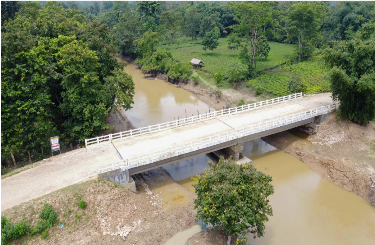
Br. No. 2/1 on Gazpuria Ali to Lukumari Demow Kinar Bongali under PMGSY Work Completed
